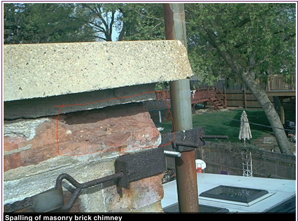
Spalling of masonry brick chimney Brick.
