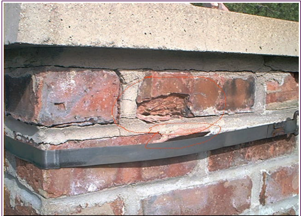
Spalling of masonry brick chimney
